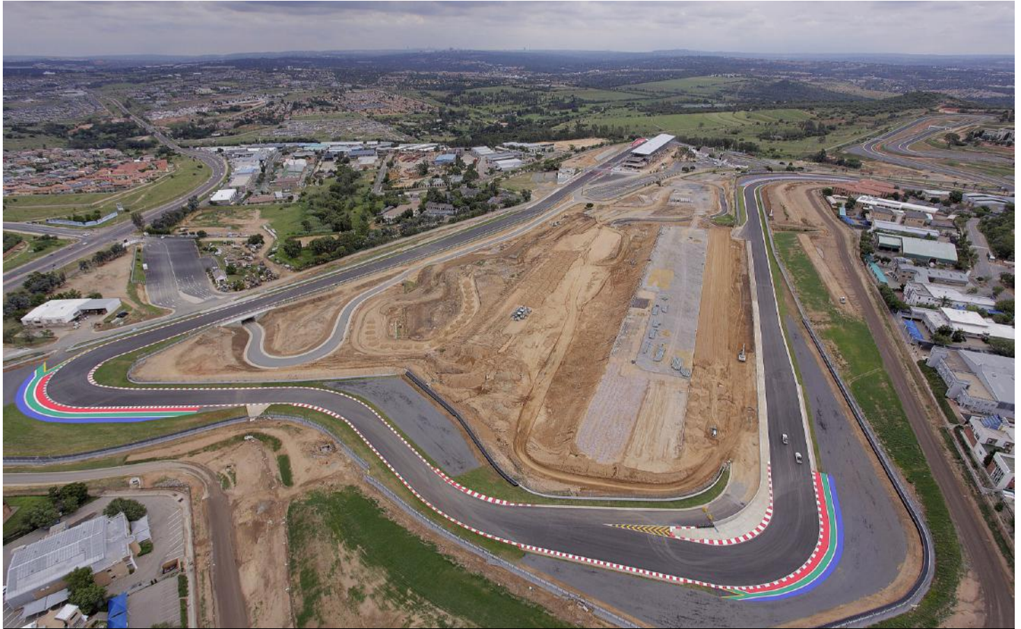
View of the circuit with Crowthorne, Jukskei and Barbeque in the foreground. Platforms and Handling Track under construction.
