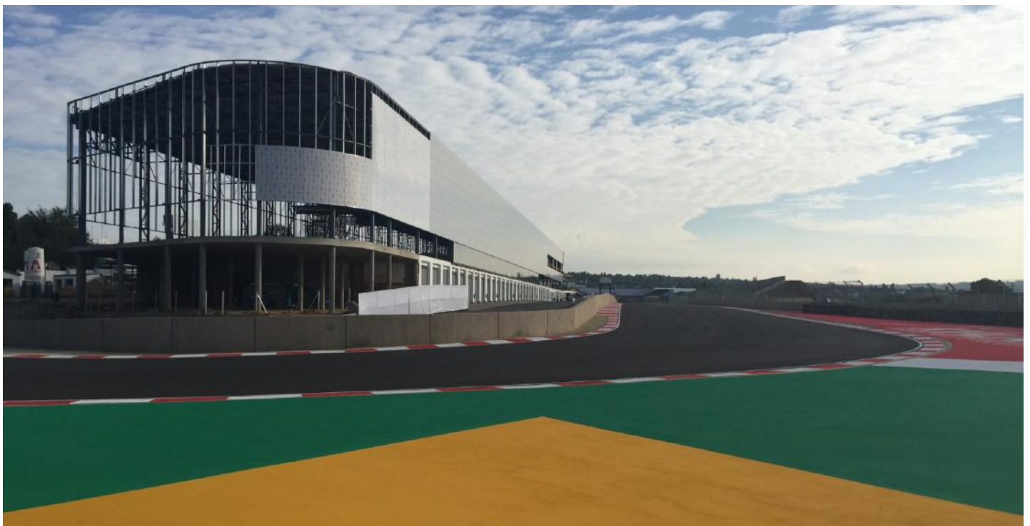
Ingwe corner with the new Kyalami Pit Building and International Convention Centre (under construction) in the background.
