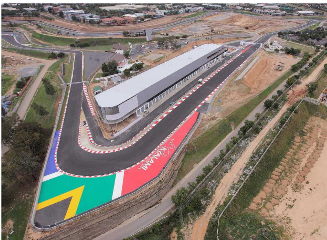
Aerial image of Ingwe corner and the impressive new Kyalami Pit Building and International Convention Centre that is still under construction.
