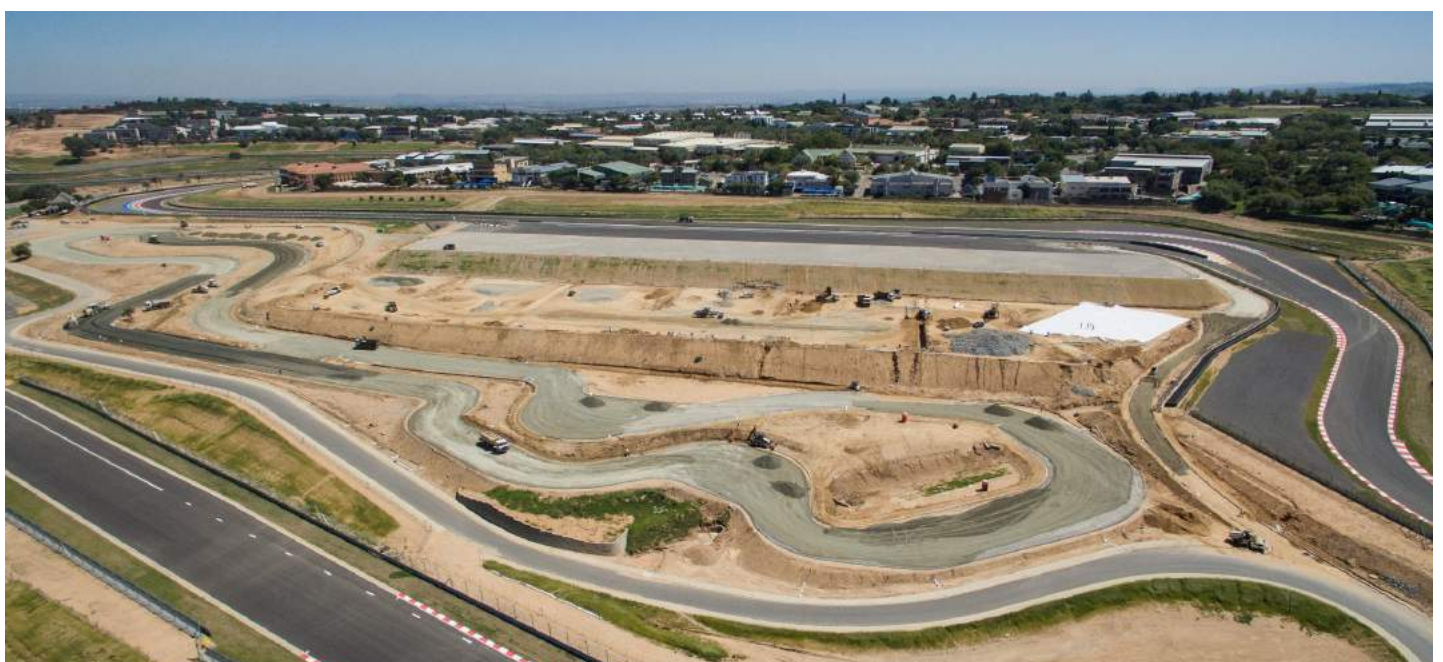
The lower section of the 1.1km handling circuit being prepared for asphalt surface. The lower platform and skidpan area is still under construction with the upper platform, now complete, visible above.
