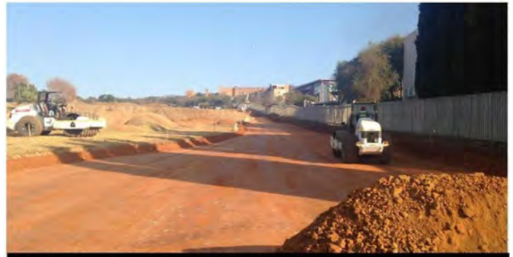
The service road is being repaired and resurfaced going up towards the 4 x 4 facility ending behind Leeukop corner.
