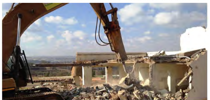
Boma 26 (Old Castrol Boma) is demolished. Most of the bomas between Clubhouse and Sunset have already been demolished.
