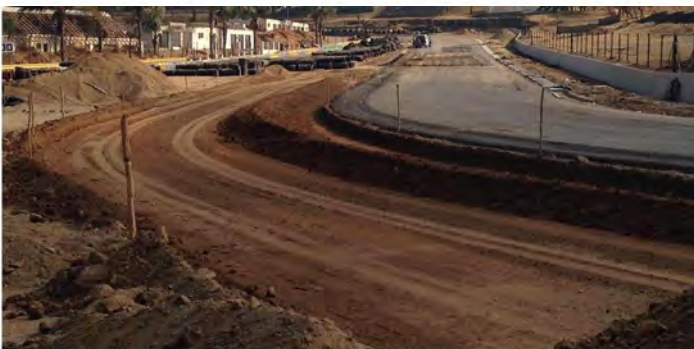
The run off area at Sunset being prepared. The gravel trap will have a section of tar run off as part of new safety upgrades.
